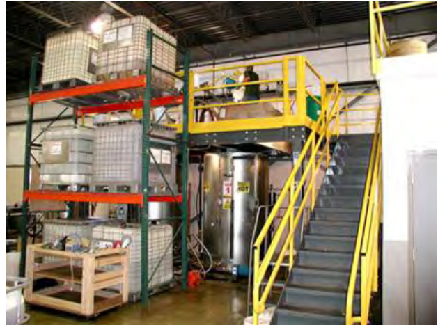
Batching Mezzanine / Batching Tanks
